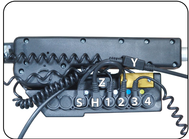
Fig. 6.2.05 – Controller with motor power cables
